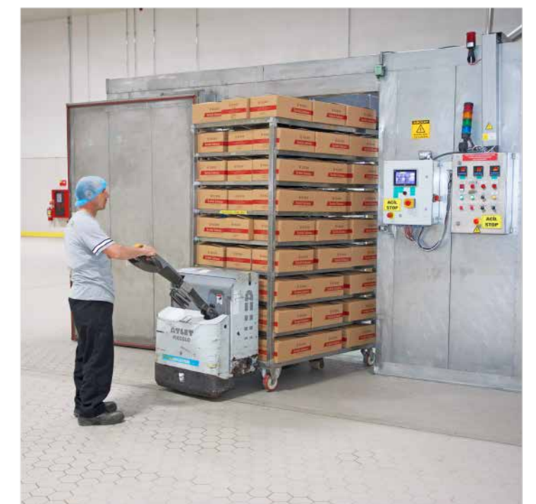
Oven treatment facilities
